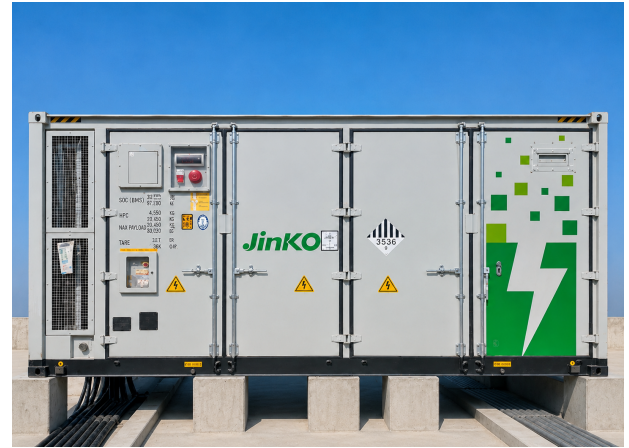
Fig. 4: PCS skid, TR1 E-house and SunTera container
