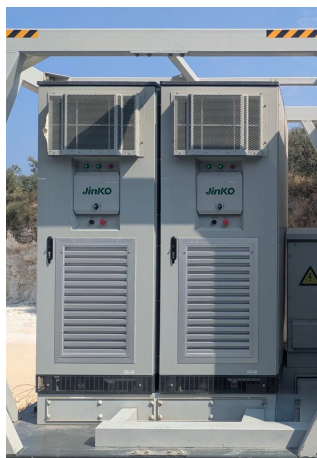
Fig. 5: PCS units inside the skid
