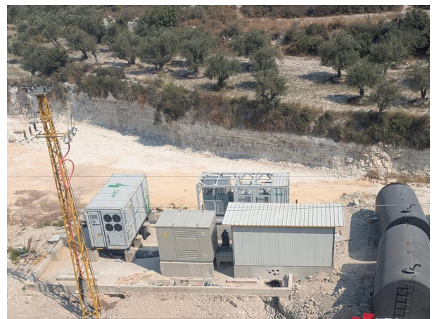
Fig. 6: Aerial view of the BESS area with the 11 kV link pole
